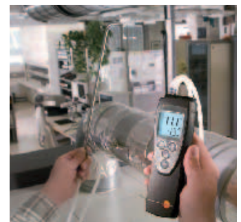
Measuring process air
